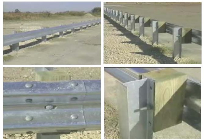
Figure 1 – Typical standard W-beam guardrail G4(1s).
